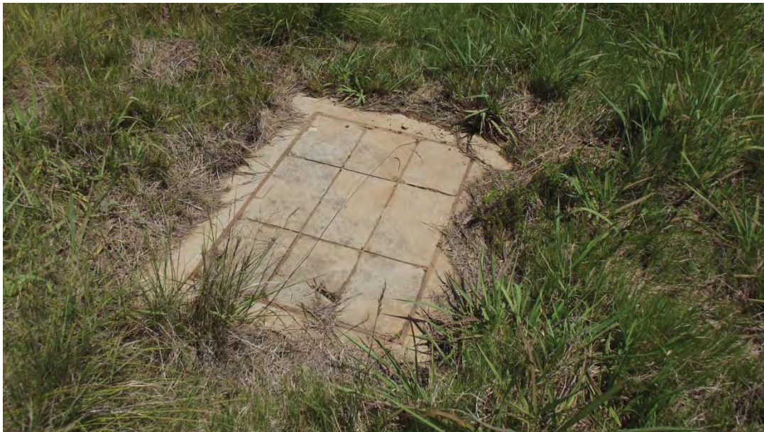
SEALED PIT 2 OFF
