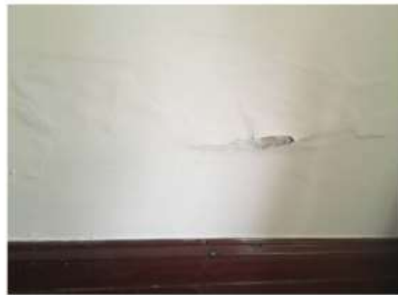
Figure 33: Room 02, evidence of damp issues
