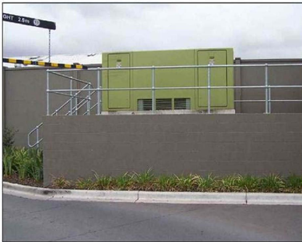
Figure 51 - Example substation raised above 1:100 flood level
