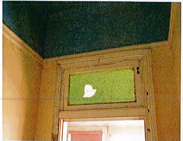
Section of architrave has been removed from the doorway at the northern end of the Cross Corridor
