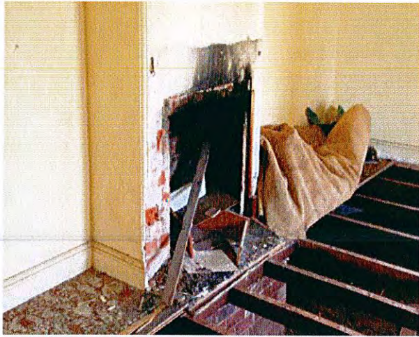
Fireplace and surrounds removed during more recent vandalism
