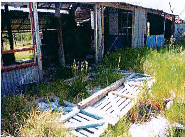
Timber frame construction with corrugated iron walls and roof. The structure is generally in poor condition
