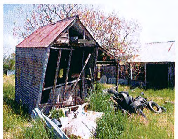
Derelict condition of Building 9
