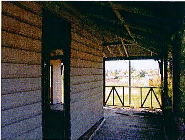
Eastern end of front verandah (VF) with doors to Living Room removed as a result of more recent vandalism
