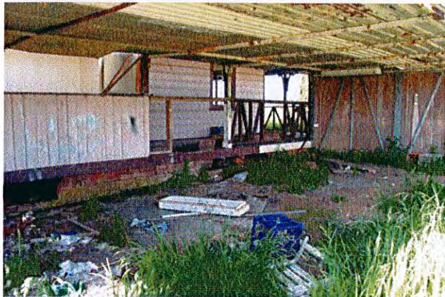
Carport on western side of house of tubular steel construction with plywood panels and clear corrugated roofing
