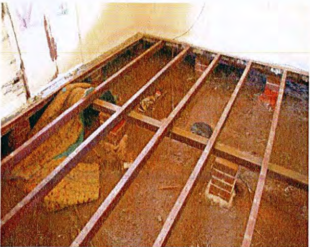
The floorboards have been removed from the bedroom as a result of more recent vandalism
