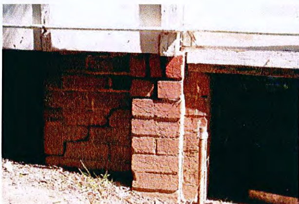
Cracking to brick piers at rear of property
