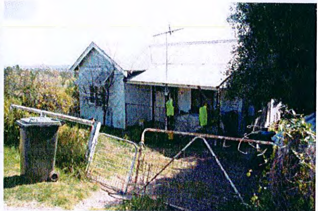
Fencing to garden and grounds of the second cottage are generally in poor condition with makeshift fencing material and gates constructed to provide some security to the property
