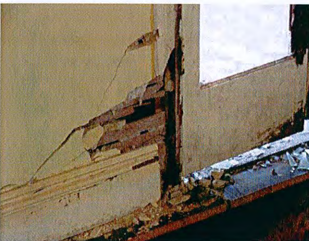
Deteriorated lathe and plaster wall, adjacent to french doors. Also of note is the clean edge where the timber flooring has been removed from the bedroom as a result of more recent vandalism.
