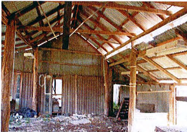
Detail of roof structure and pole construction of main section of Building 8
