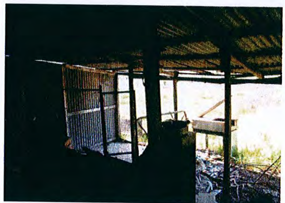
Internal layout Building 6 with profiled corrugated sheeting on walls and roof. Of note is the timber pole and timber framed construction
