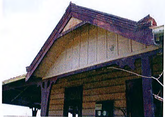
Detail of gablet on southern elevation with timber barge boards and proprietary pressed metal gable end
