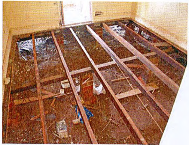
The floorboards have been removed from the bedroom as a result of more recent vandalism
