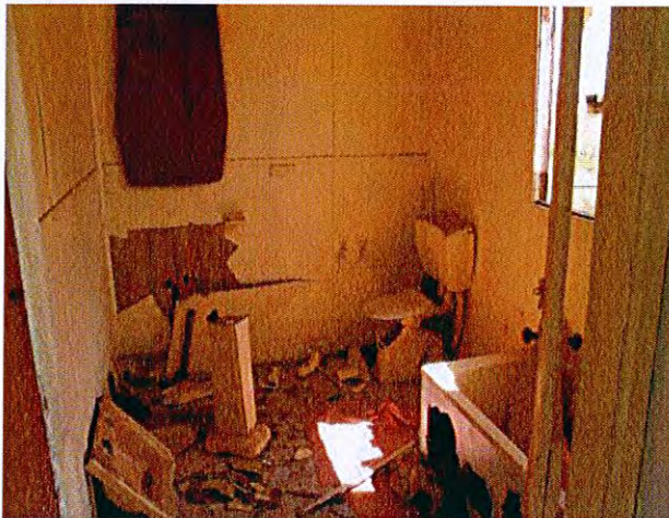
Vandalised bathroom. Of note is are the relined fibro walls with old vertical boards behind
