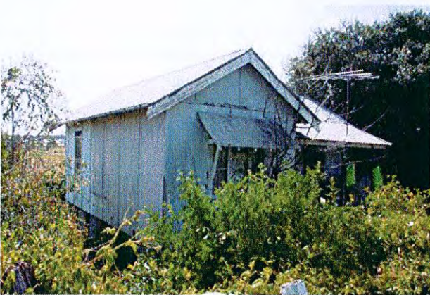
Timber frame construction, fibro sheeting to walls and corrugated iron roofing material. Also of note is the remnant garden which has also suffered from neglect
