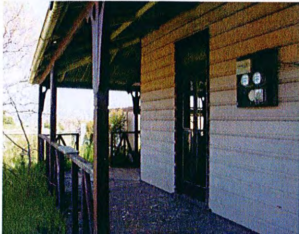
Timber verandah on southern elevation with simple painted timber balustrade and supports
