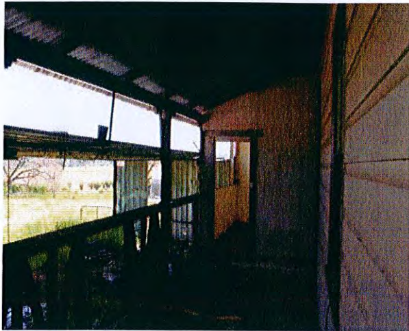
Car port and western verandah with timber balustrade, timber floorboards, and doorway through to sleepout (Bdm 3)
