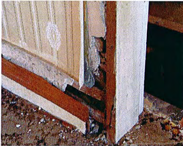
Deteriorated lathe and plaster wall behind more recent plasterboard wall which has been covered in wall paper
