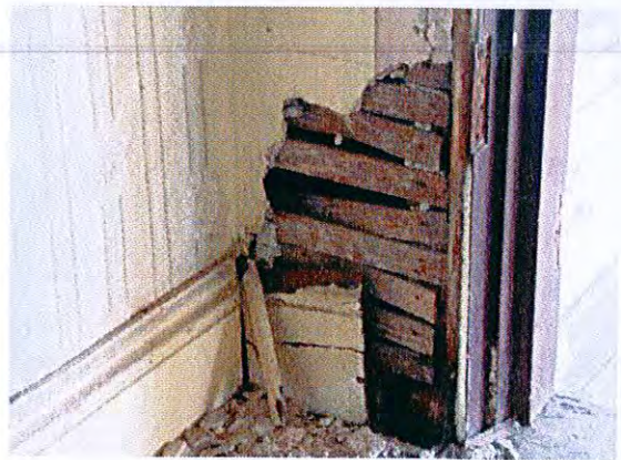
Deteriorated lathe and plaster wall in the Cross Corridor adjacent to doorway to Rear Verandah
