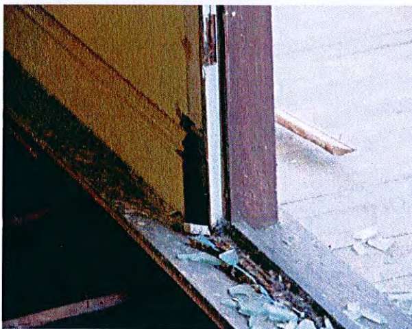
Damage to architraves and missing floorboards
