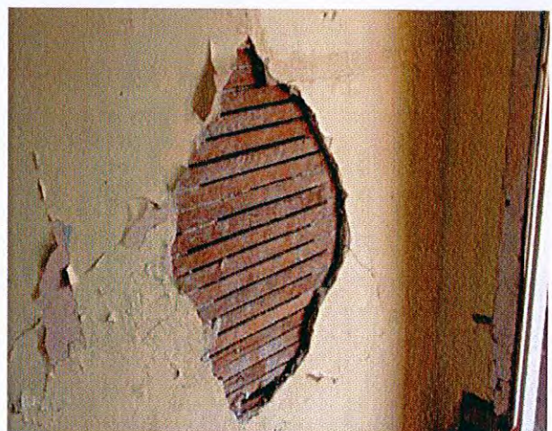
Deteriorated lathe and plaster wall
